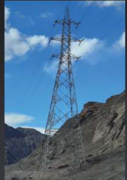
66 KVA Transmission Line, Ladhak
